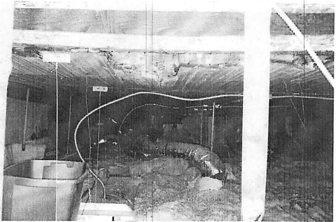
STRUCTURAL DAMAGE TO CEILING ABOVE COUNCIL CHAMBERS
